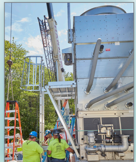
eco-ATWB-H Closed Circuit Cooler installation
