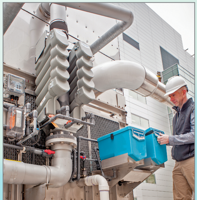
Smart Shield® Factory-Mounted Water Treatment System
