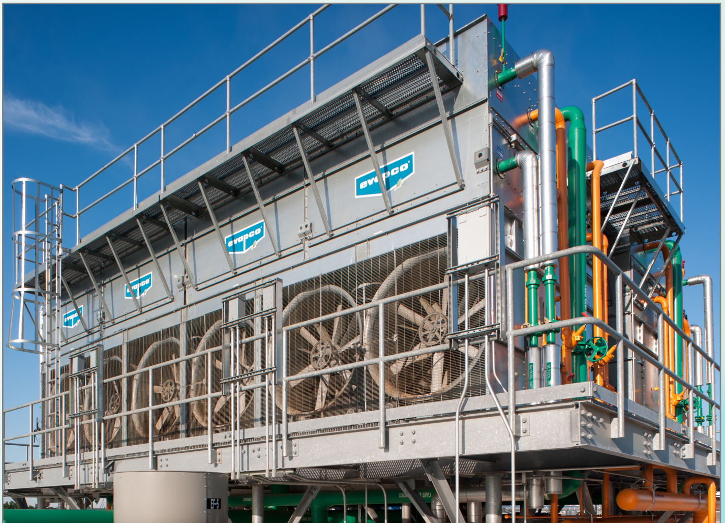
PMC-E Evaporative Condenser with external service platform.
