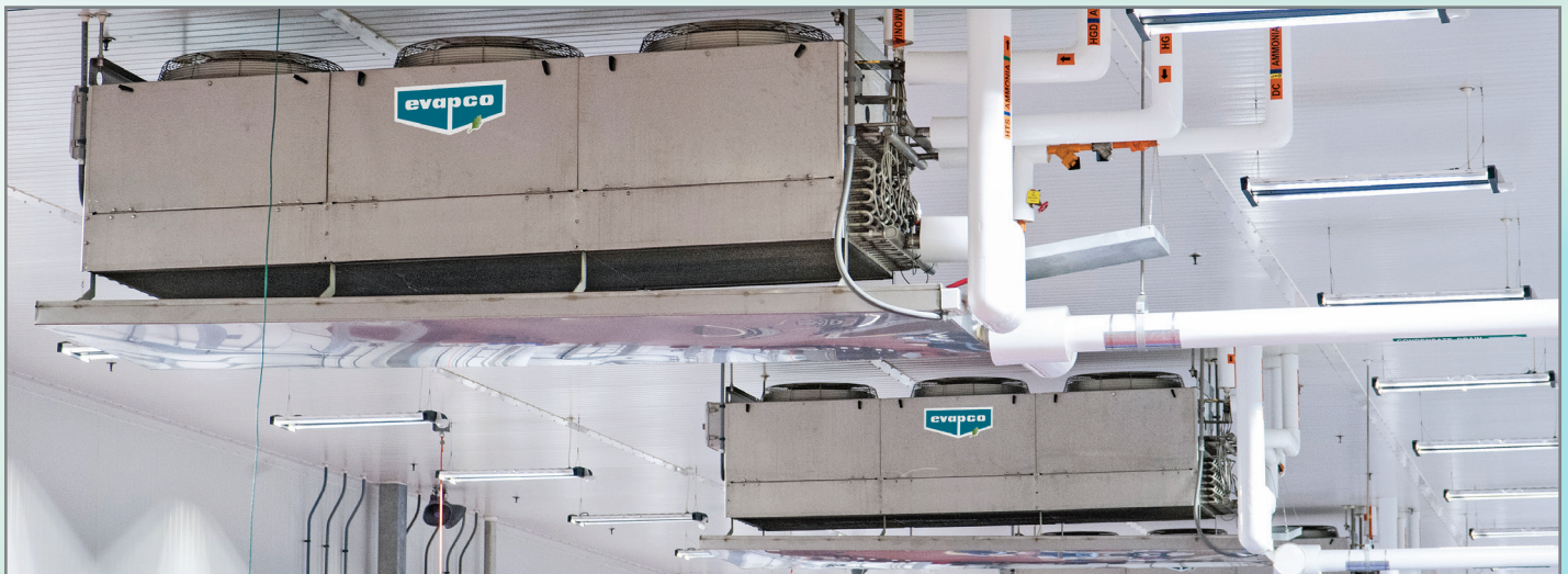
SSTWE Work-Room Evaporators
