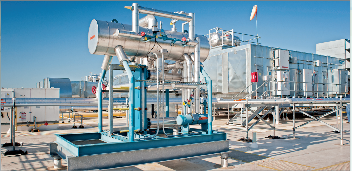
RVS MPC Chiller Package
