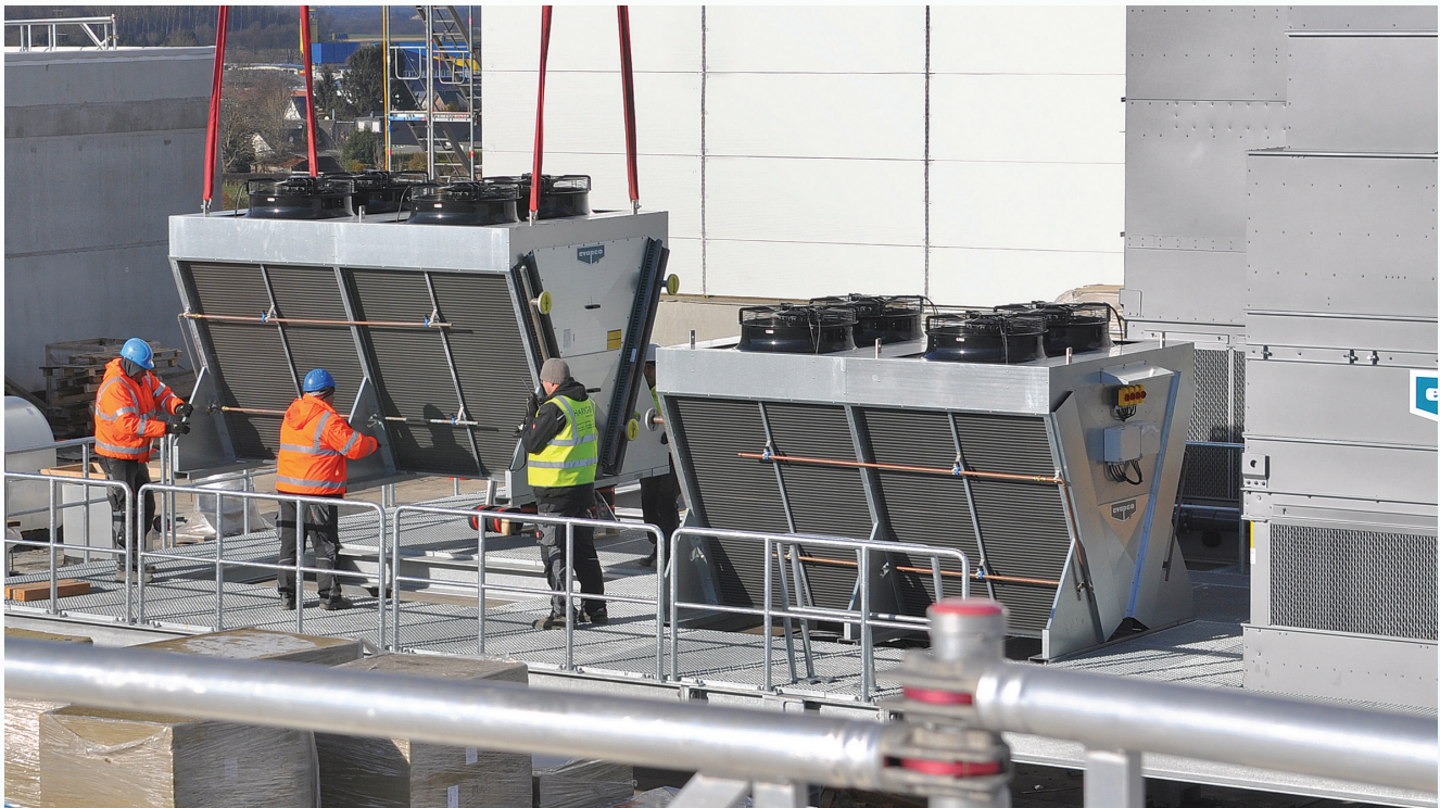
EVAPCO Air Solutions V Series, Germany
