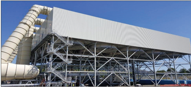
Two condensers, one structure
